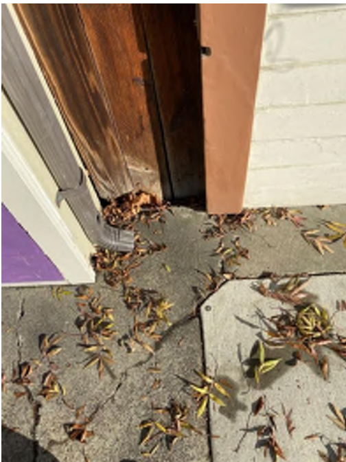
Above: Example of a Nail and Tin set in concrete sidewalk. Also referred to as a Nail and Tag . Often abbreviated as N&T .
