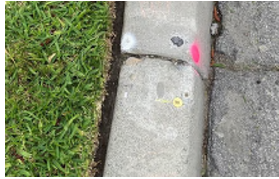
Above: A new tag and tack set in lead on the top of a concrete curb. Approximately 3/4" in diameter.
