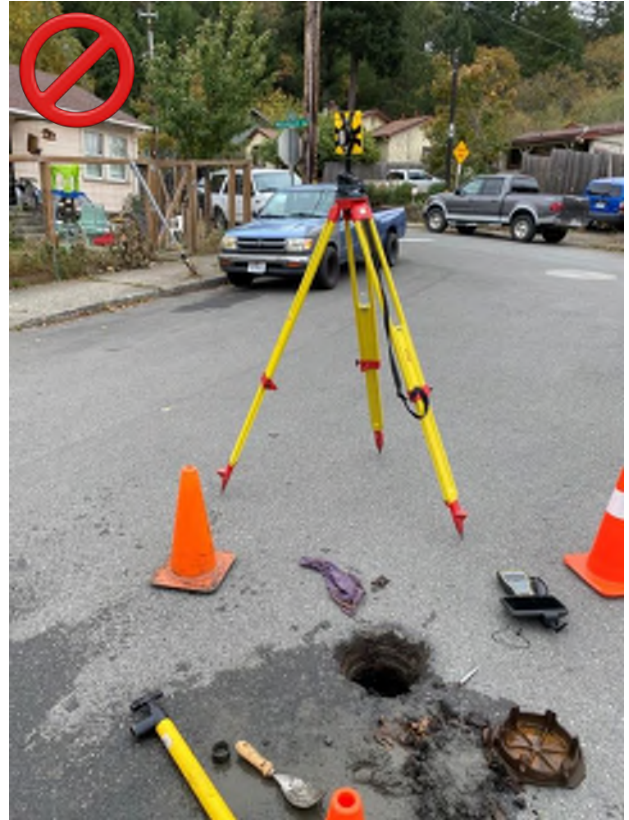
Above: A monument well that was buried beneath an asphalt overlay.
