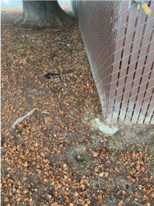
Above: 1" diameter Iron Pipe buried below the surface. Iron Pipe is often abbreviated as IP
