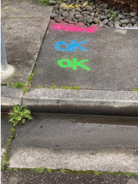
Above: Example of USA markings on a construction site. Notice the survey monument at the top of the picture.
