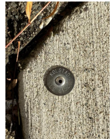
Figure 5: Close-up of Figure 4. Approximately 3/4 inch diameter
