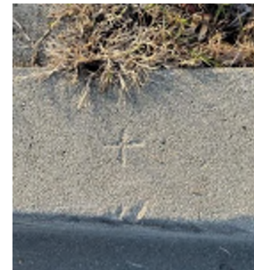
Figure 10: A chisel cross (circa early 1970s) in a top of curb likely set to denote the boundaries of lots in a subdivision. For perspective the curb is 6 inches wide.
